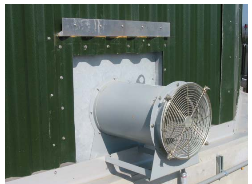
Four 2-speed tubeaxial fans were provided to ensure proper airflow was maintained through the Sessil media bed.
