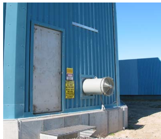
Four 2-speed tubeaxial fans were provided to ensure proper airflow was maintained through the Sessil media bed.
